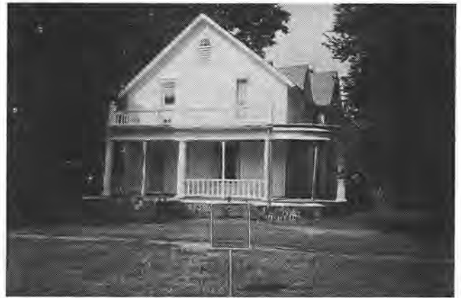
Adopted granddaughter of Oscar Cather (brother of G. P. Cather, One of Ours, and son of George Cather), Sayra Wagner, has done exterior repair, roofed, and painted the Charles Cather house, located on Sixth and Seward in Red Cloud. Renovation of the porch and interior continues. The Cathers lived in this house from 1904 until Mrs. Cather's death in 1931. — Photo by Pat Phillips
